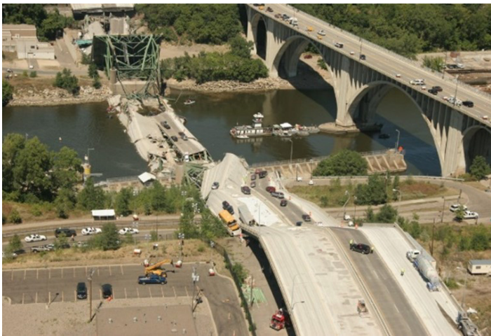
Figure 1: The I-35W Mississippi River Bridge, which catastrophically failed during the evening rush hour on August 1, 2007
